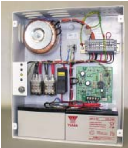
Group Control Panel
